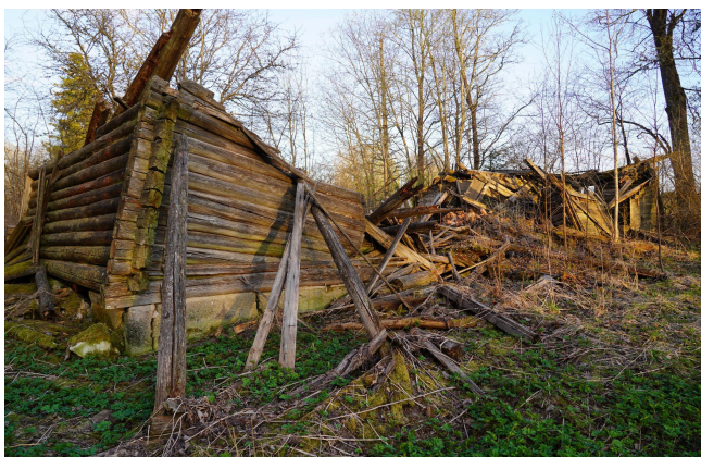
Fig. 15. The process of a modern country house's destruction. The main part of the structure collapsed inside the house and the roof details have not survived to the present day. Jõgeva County, Estonia (Photo: I. Khrustaleva).
