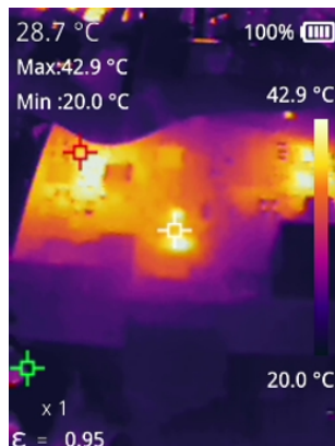
Figure 22: Thermal camera image of the EPS after the aforementioned fix
