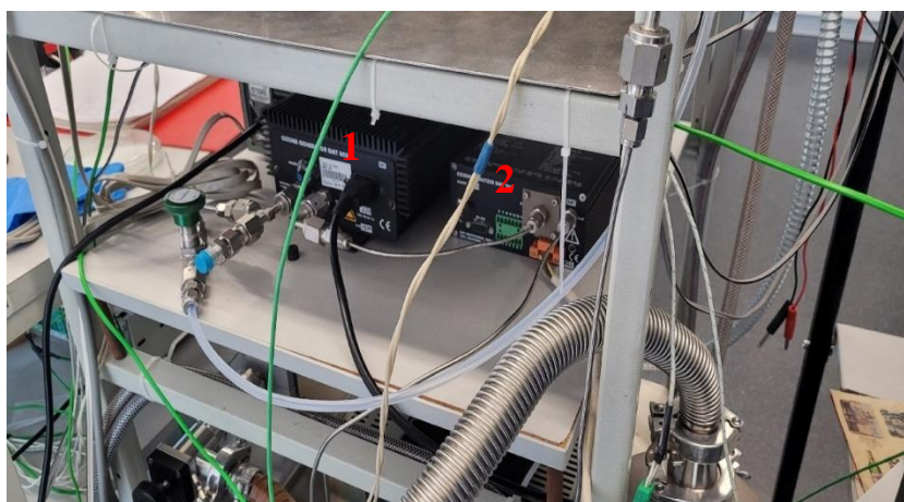
Figure 35. Back view on Ozone generator (1) and analyzer (2).
